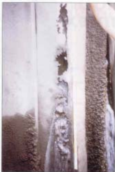
Figure 4 Removal of marine growth and rust deposits, along with thorough abrasive cleaning, is necessary to avoid the damage done by underwater corrosion. The steel piling has then to be restored and perforations filled and welded prior to applying the HUMIDUR® system.
