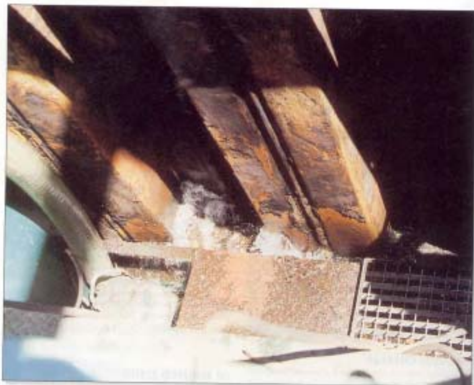
Figure 2 Underwater corrosion is covered by a multitude of mutually inertive processes
