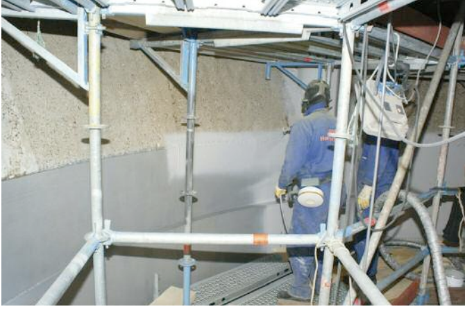
Left, from top to bottom – Application of the first layer of Humidur on the vertical armouring of the intake tower
