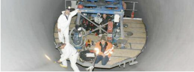
Control of the sandblast cleaning in the pressure shaft, final control of the cleaning (adhesive tape test) before release for coating application
